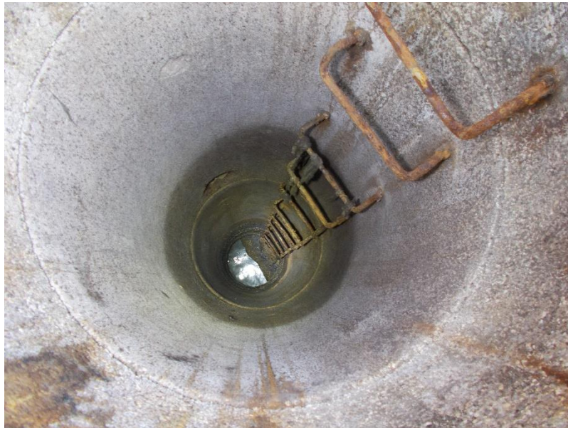
Tylehurst Lift Station Wet Well
